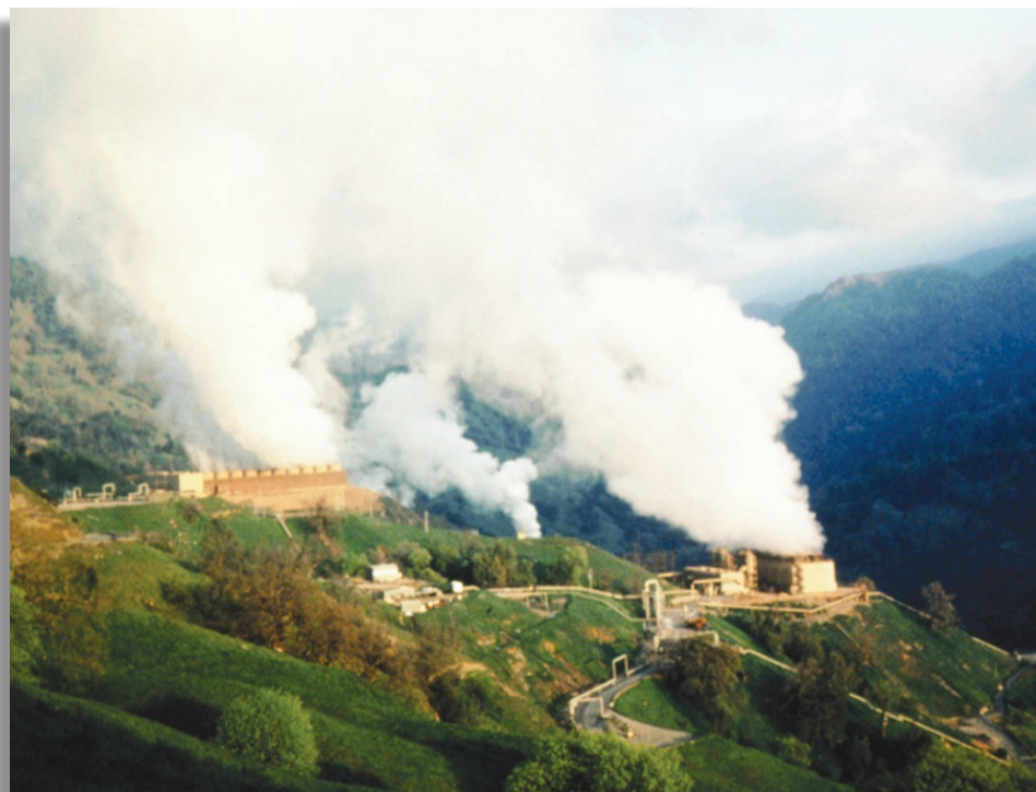
Geothermal power plants at The Geysers in northern California. Currently, the United States has an installed and utilized power production capacity of more than 2,500 Megawatts-electric (MWe) from geothermal plants located in Alaska, California, Hawaii, Idaho, Nevada, and Utah. (USGS photograph by Julie Donnelly-Nolan.)
