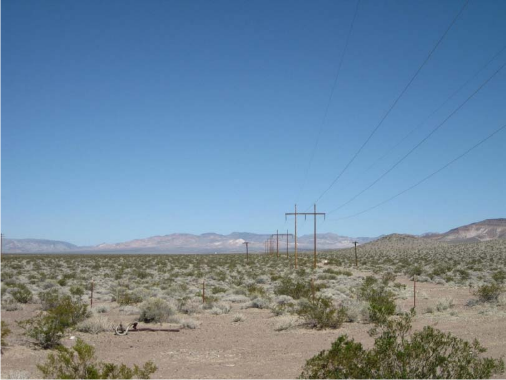
Figure 8. Typical Transmission Line Towers
