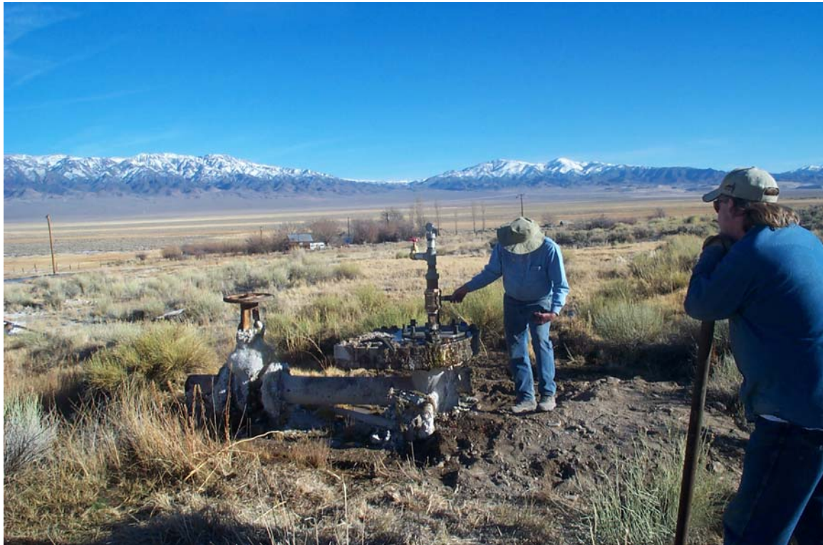
Old geothermal well. Cleaning main stainless steel slab valve and installing small valve and access port
