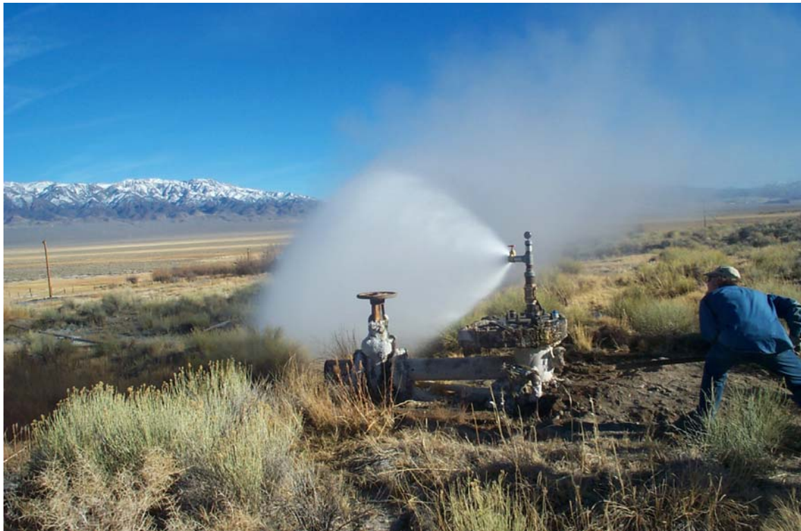
Darrough geothermal well – small 2" valve and pressure gauge
